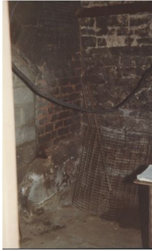
Fig 2 Blocked off passage way on the charnel house
