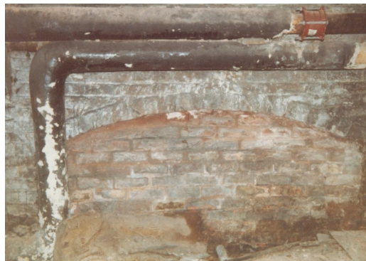
Fig 4 Blocked arch by the boiler in the charnel house
