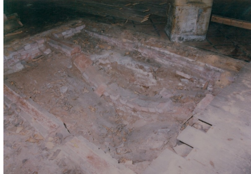
Fig 6 Collapsed brickwork in south block
