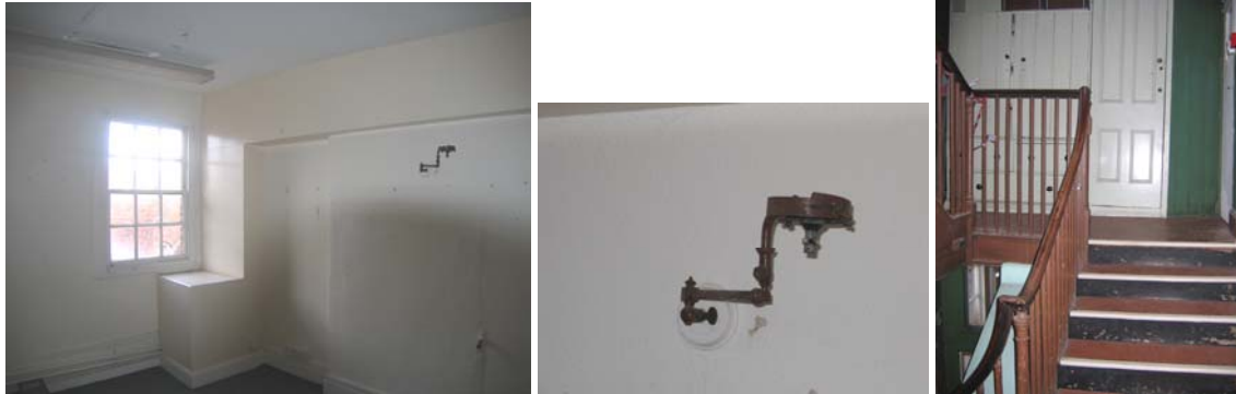
2F-04; gas bracket 2F-04; Staircase
